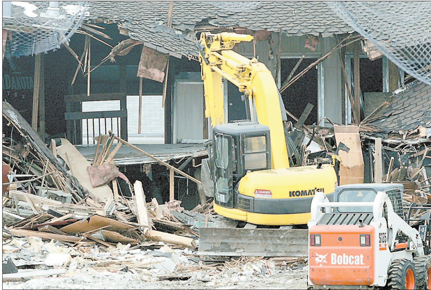
The Pressbox, already weakened by a fire in September 2008, was no match for heavy demolition equipment Monday afternoon. Chad Gruenwaldt, owner of the Vermillion tavern, and the city of Vermillion reached an agreement last month calling for the demolition of damaged structure. (Photo by David Lias)
