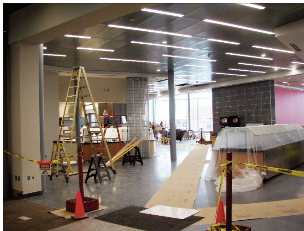
Some of the expanded portions of the Muenster University Center are now visible to visitors. Passersby have been able to glimpse the new sections of the building for at least a week. The completed facility will feature expanded seating and national restaurant options, such as Chick-fil-A, Qdoba and Einstein Bros. Bagels, the last of which has been open for some time. The 31,000 square foot expansion is budgeted at $11.6 million, and university officials said last summer that they hoped it would be open by the beginning of the 2014 spring semester. The original MUC building opened in February 2009, and expansions of it have been discussed since USD President James Abbott's State of the University address in 2011.
