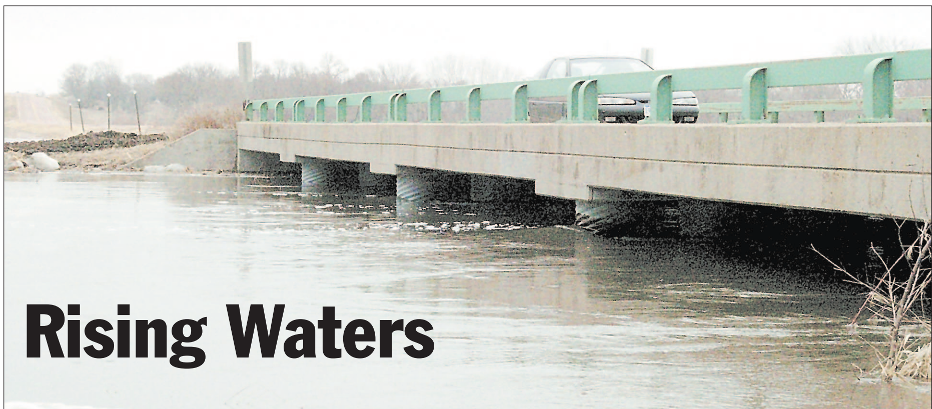
A car slowly drives over the bridge that spans the Vermillion River on 306th Street, commonly known as the Volin Road, Monday afternoon north of Vermillion. A portion of the road near Highway 19 was closed later in the week as water continued to rise. (Photo by David Lias)
