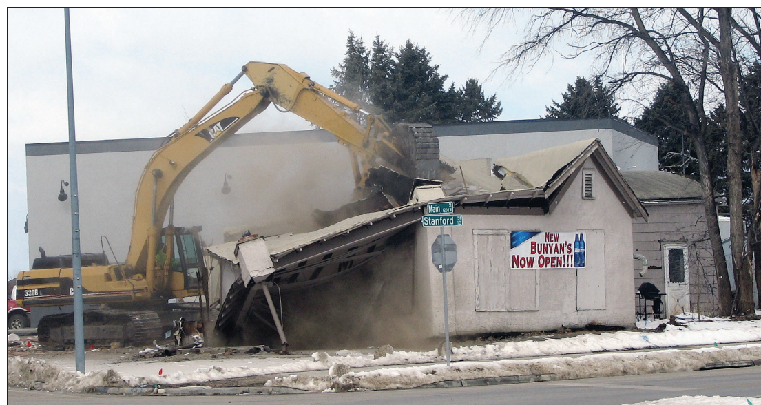
The old Bunyan's was demolished the morning of March 1, taking away one of Vermillion's long-time watering holes. A new Bunyan's opened on Dec. 22 in a building constructed behind the old one. The new building also houses the Chop Shop, a hair salon.
