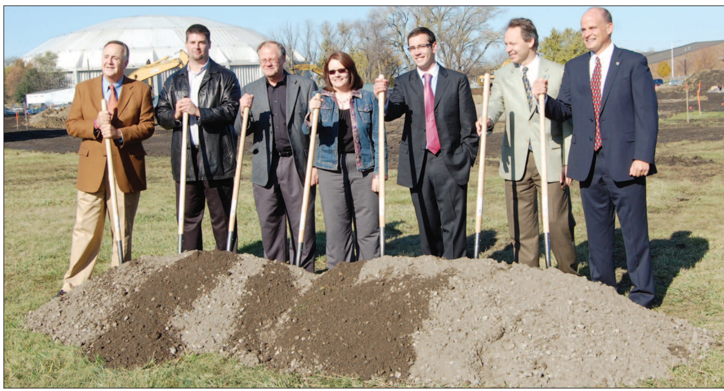
Dig in! Monday's program featured groundbreaking for the new University of South Dakota wellness center, but construction is already under way. Taking a turn with shovels are (from left) USD President Jim Abbott; Eric Schuler, project manager with the Henry Carlson Company; Paul Klein with RDG Planning and Design; Kirsten Company, USD associate dean of students; Ryan Budmayr, former USD Student Government Association (SGA) president; Rich Van Den Hul, USD vice president for finance and administration; and USD athletics director Joel Nielsen. Company and Nielsen co-chaired the wellness center planning committee. (Photo by Randy Dockendorf/Yankton Media Inc.)
